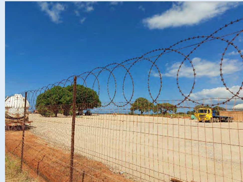
Fencing Wire mesh fencing of 2 mtr height with razor wire on top
